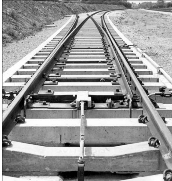
Photo 2.16 Modern catch point. (Pandrol Rail Fastenings Ltd).
