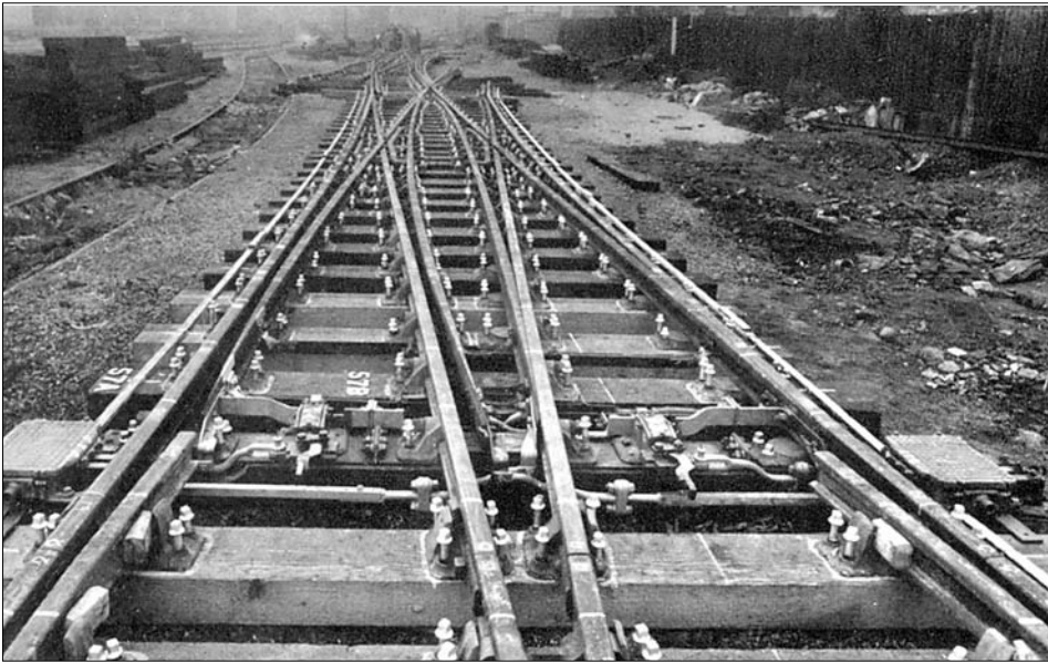
Photo 2.11 Double slip switch under construction. Note fittings for detection and locking have been pre-attached. (Balfour Beattie Rail Eng.).
