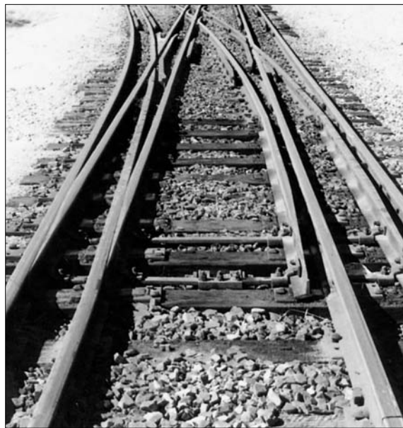
Photo 2.22 Triple gauge turnout at Gladstone, South Australia. (Pandrol Rail Fastenings Ltd).
